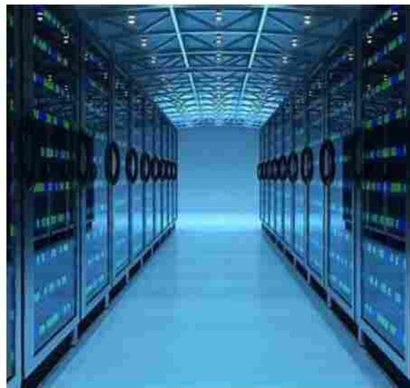
Tier III+ and Tier IV ready digital infrastructure
