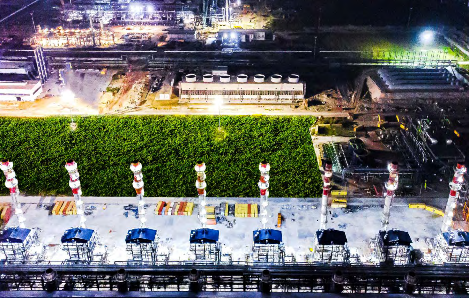
Aerial view of Heat Recovery Generator for Captive Power Plant
